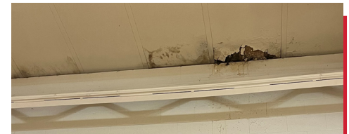
Deteriorating Gymnasium Ceiling
