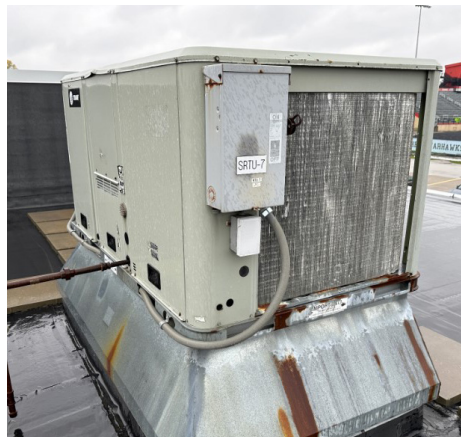
Failing HVAC System
